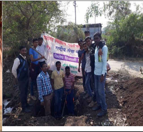
NSS Volunteers along with NSS programme officer Digging the Soak Pits in village ChikhurdaTq. Dist. Latur
