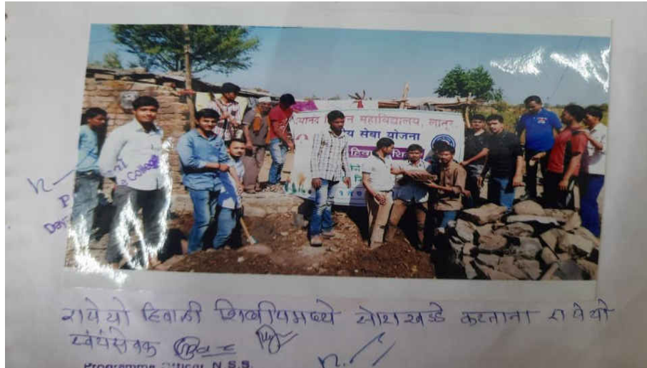
N.S.S. Volunteers Digging The Soak Pits During The NSS Camp at Chikhurda on 01-07.2017
