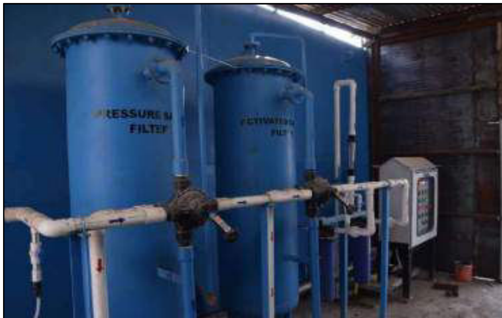
Figure 11: Sewage Treatment Plant
