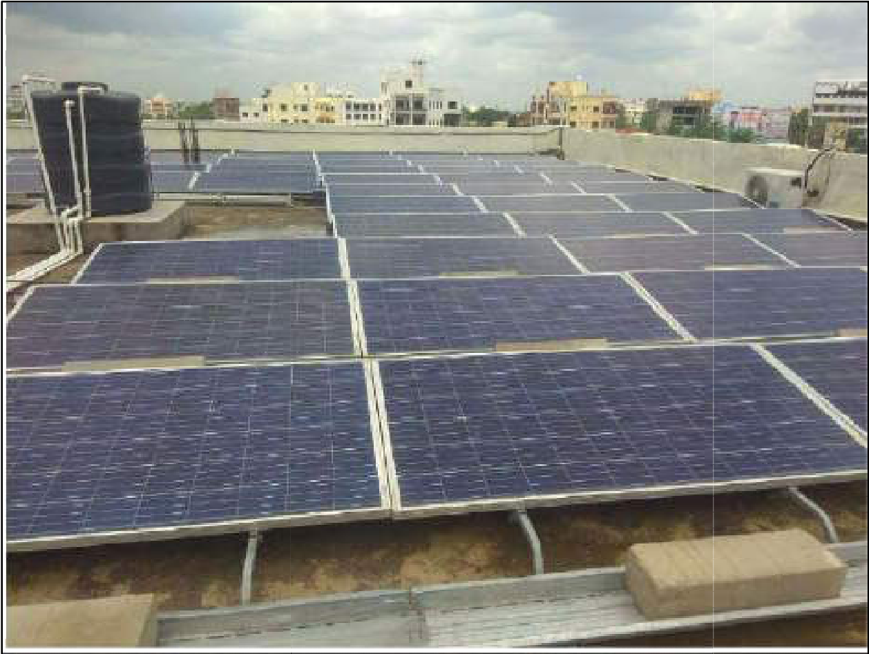
Figure 13: Solar Panels On Rooftop
