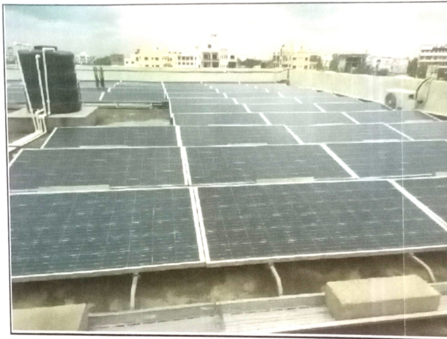
Figure 13: Solar Panels on Rooftop
