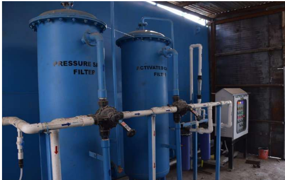
Figure 11: Sewage Treatment Plant
