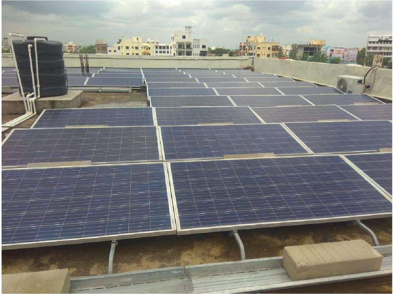
Fig No 13: Solar Panels On Rooftop
