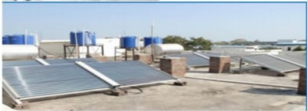
Solar Panel water Heater In Girls Hostel
