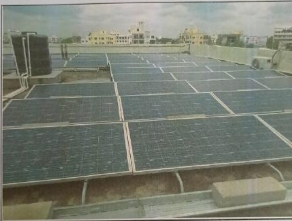
Fig No 12: Solar Panels On Rooftop
