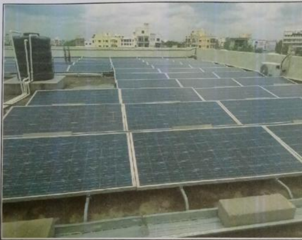
Figure 12: Solar Panels on Rooftop
