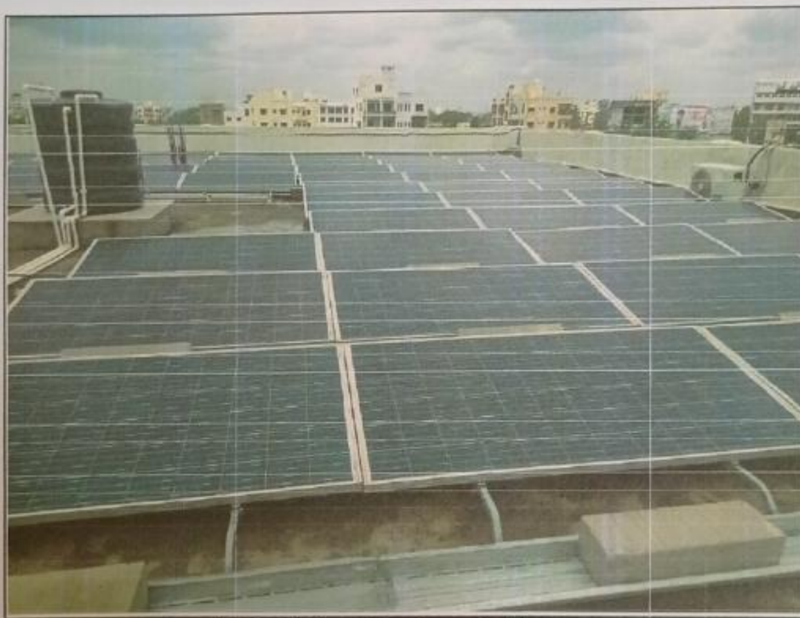
Fig No 13: Solar Panels on Rooftop
